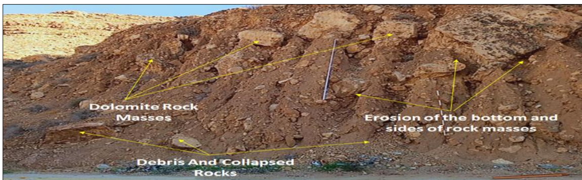
Figure 9: Section of the Slope Affected by Gully Erosion
